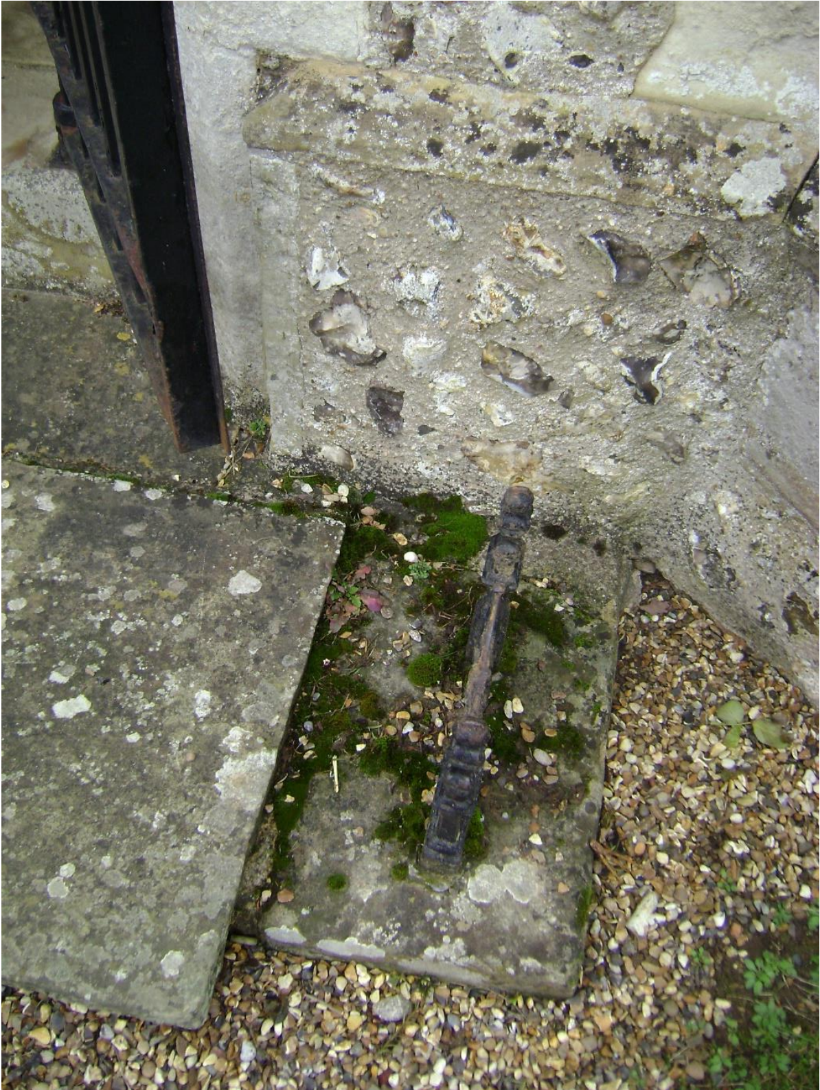
The stone slab bearing the boot-scraper by the main porch is particularly mossy. It is probably quite damp and gets occasional loading of nutrients!
