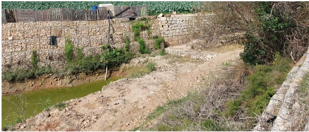
Fig 2. Valley bed and understory scraped off in a valley rehabilitation project at Wied il-Fiddien
