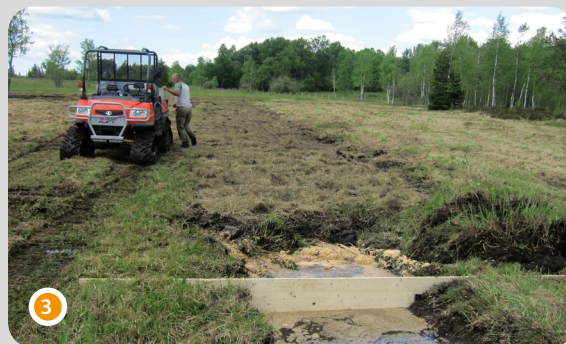
Step 3 in the ditch neutralisation: covering the sawdust with peat from the clearance of mineralised peat
