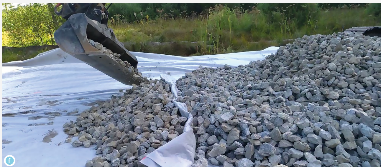
Installation of a sheet of low-permeability geotextile. Embedded every five metres, these sheets prevent the water from circulating longitudinally in the filling material (limiting its draining effect) and direct it preferentially to the other side of the road, towards the downstream peat
