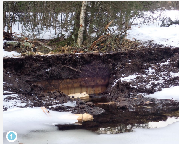
The water passed underneath the fencing, which was not anchored in the watertight substrate, re-emerging by artesian flow at the weak point created by the hollow from where the peat was taken
