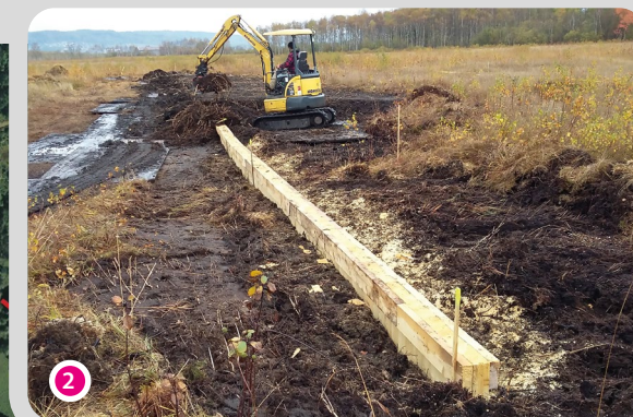
Covering a single wooden fencing dyke with peat. To avoid creating draining ruts in the ground, the excavator is working on plates
