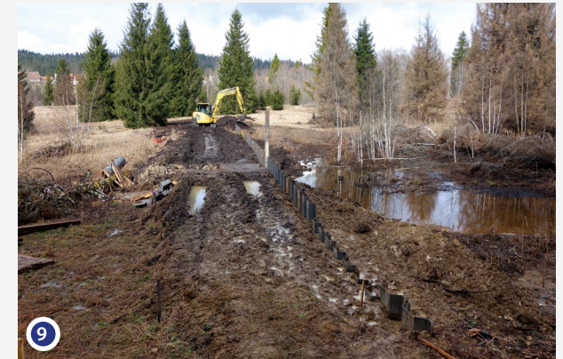
Reinforcement of the dyke by installing a curtain of steel sheet piles. This would then be covered with peat and become vegetated.
